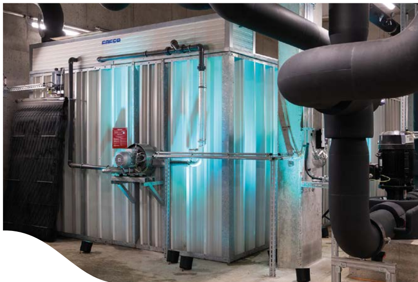
The ice storage facility at MedUni Campus Mariannengasse: highly efficient chillers cool water to five to six degrees Celsius, which is distributed throughout the building to provide pleasant cooling.
